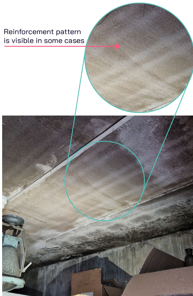
Figure 17: Signs of excessive moisture content. (Source: MTC. With permission of Airedale general Hospital)
