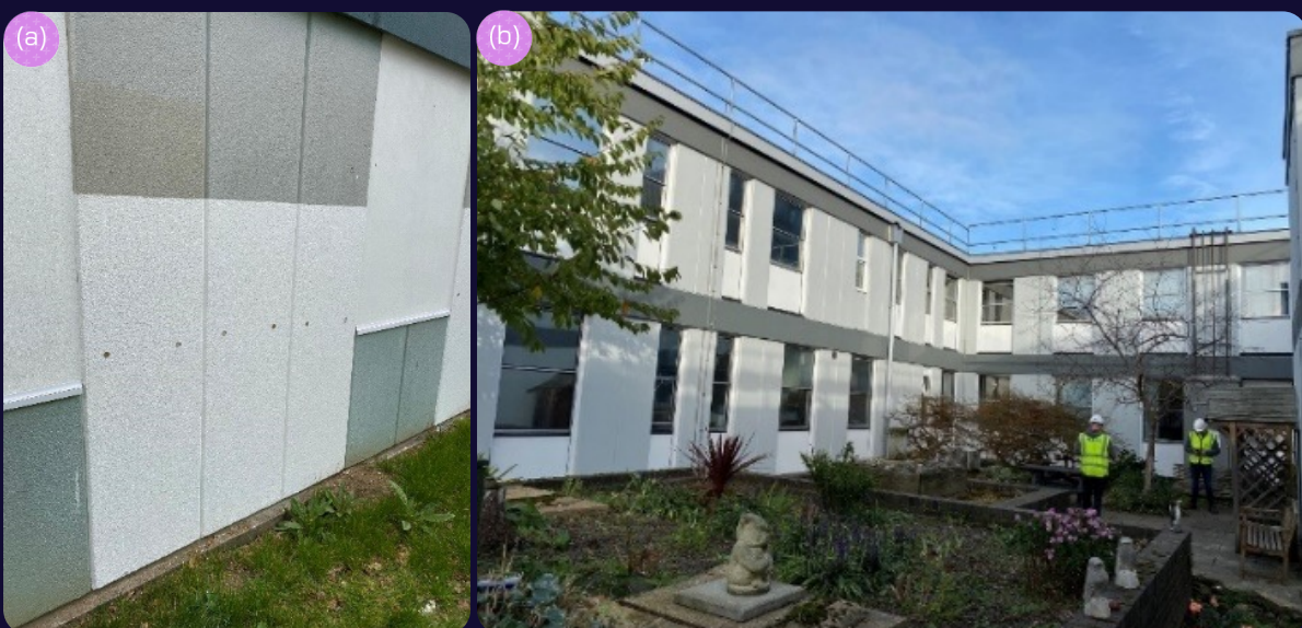
Figure 70: Remedial work on RAAC Panels, (a) close-up of effected RAAC panels, (b) impacted structure
