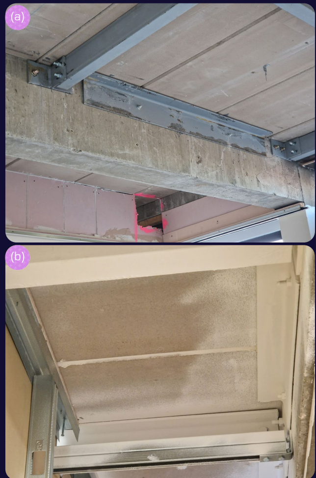
Figure 79: End bearing strengthening in (a) large width hospital room, (b) hospital corridor. (Source: MTC. With permission of Leighton Hospital)
