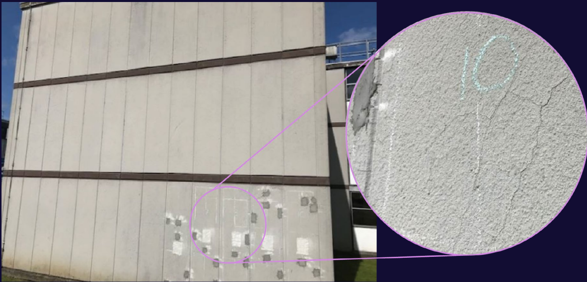
Figure 69: Evidence of localised cracking and deterioration
