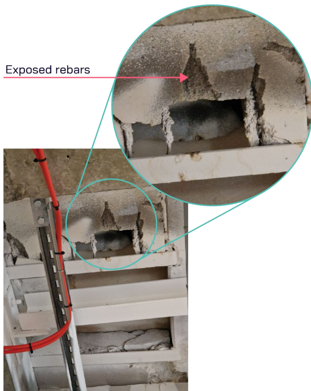
Figure 21: Exposed rebar due to poor workmanship (Source: MTC. With permission of Leighton Hospital)
