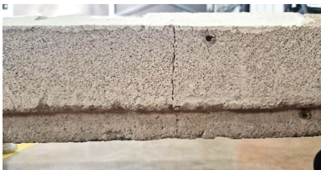
Figure 15: One of the sectioning cracks located 30cm along a RAAC plank. Source: MTC, 2023.
