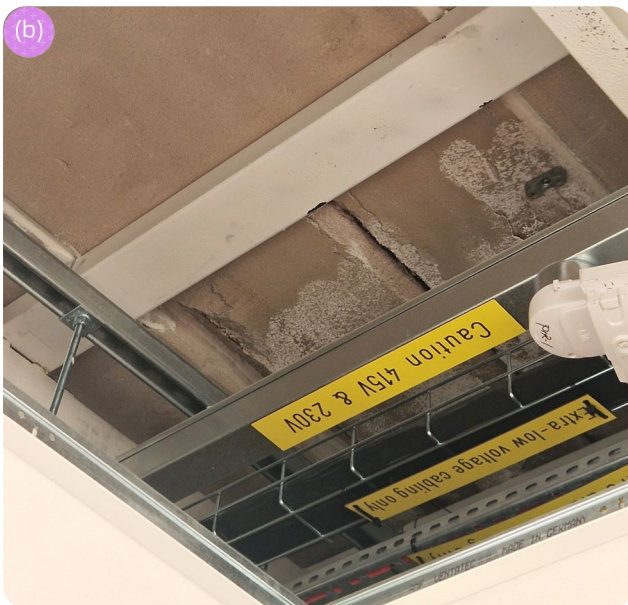
Figure 67: (a) Planks affected by an inactive leak and efflorescence around the bearings. The position of the rebars is drawn onto the surface consequently (Source: MTC. With permission of Airedale General Hospital). (b) Plank affected by an inactive leak, efflorescence, and corrosion with the spalling of the cover (Source: MTC. With permission of Leighton Hospital).
