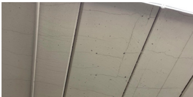
Figure 14: Transverse and longitudinal cracks in RAAC roof planks [10]
